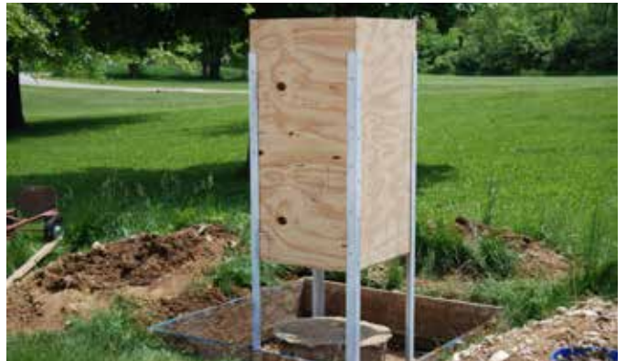
The base section in the hole, showing the form for the concrete, the depth of the hole and the old concrete from the basketball hoop.
