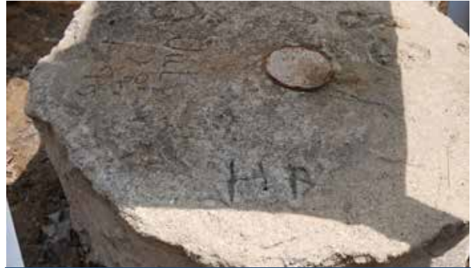
The start of digging away the dirt, rock, etc. around the concrete where the old basketball hoop had been but was cut down.
